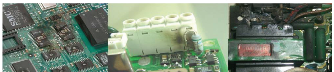
Burn-out of the electric devices due to surge
